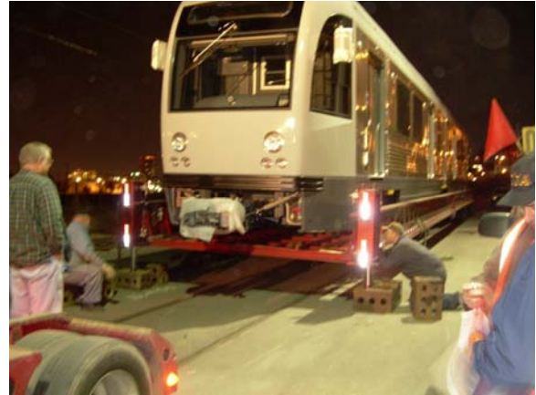
Steel blocks used for leveling hydraulic system to lower the trailer to the final height of 6 inches.
